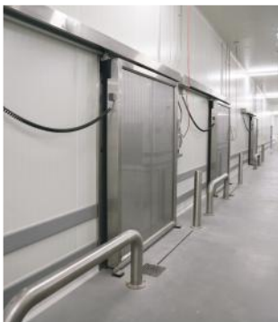
Electrically Operated Doors
