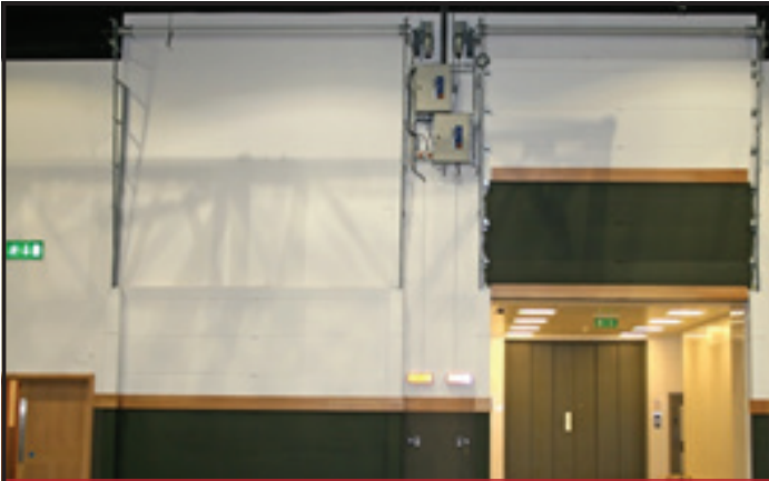
Vertical Soundslide – CCD, Dublin, Ireland
